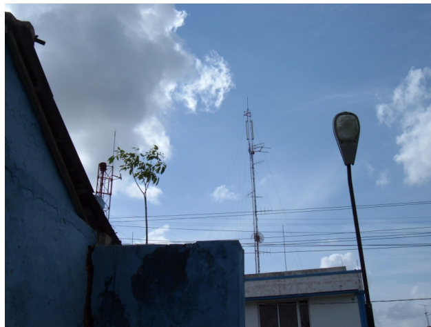
Figure 7.9: Tower in the Telephony Center of Artemisa where WiMAX Antenna has been placed
