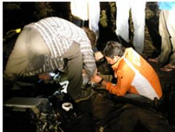
Joint box(Connecting cables)
