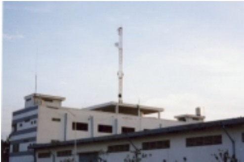
PHS Cell Station at Canadia Industrial Park
