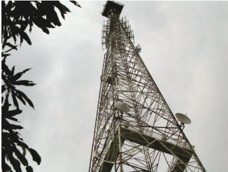
Main transmission site
