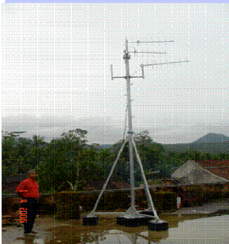
The antenna installed in the roof of the building, both for voice and broadband
