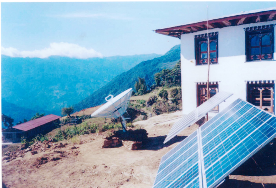
Solar panels and VSAT antenna in Sombeykha
