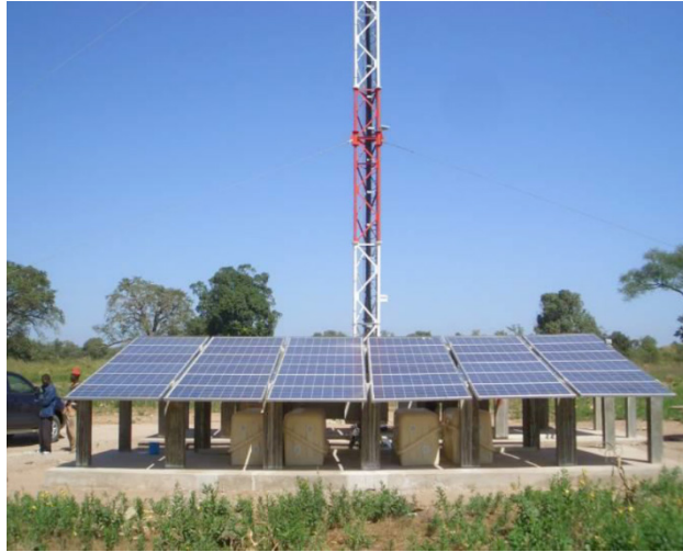
Figure 12: Solar station at a mobile network site in Senegal
