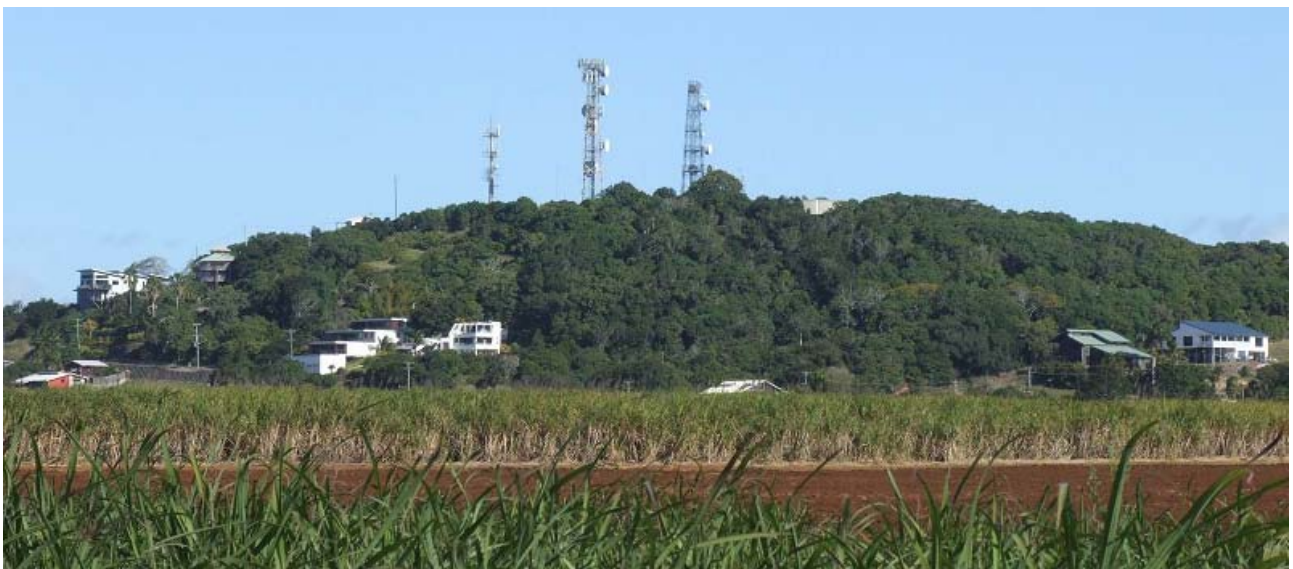
Base station at Sloping Hummock, East of Bundaberg
