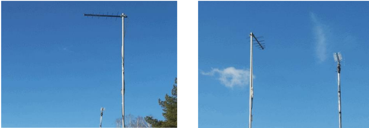
FIGURE 9 Positions of TV broadcasting receive antenna and fixed wireless broadband access system transmit antenna
