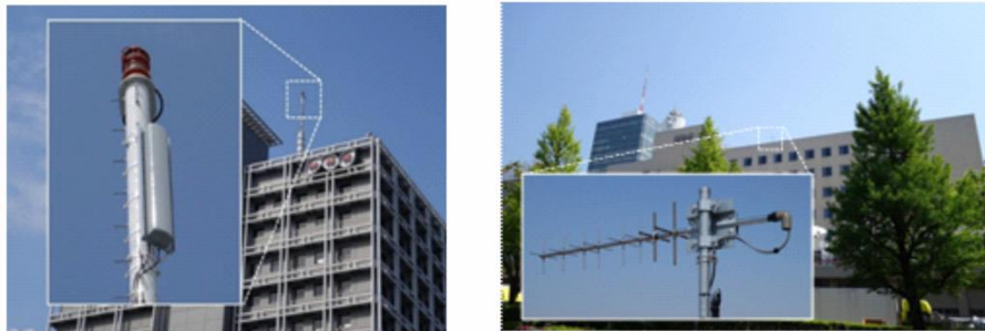
a) Transmission antenna
