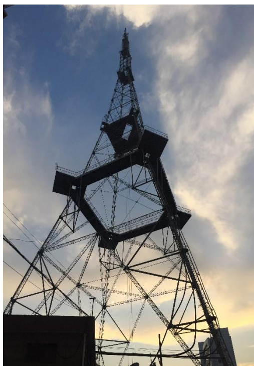
Transmission station antenna
