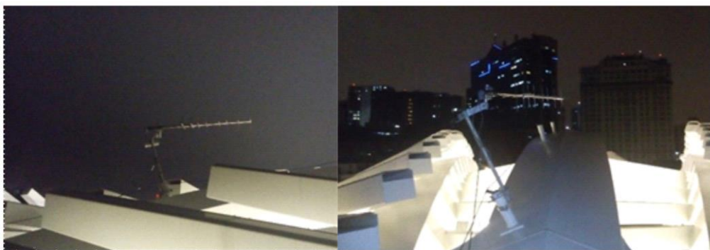
Reception station antenna
