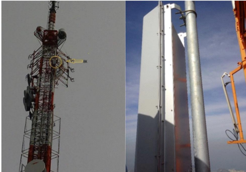
Transmission station antenna
