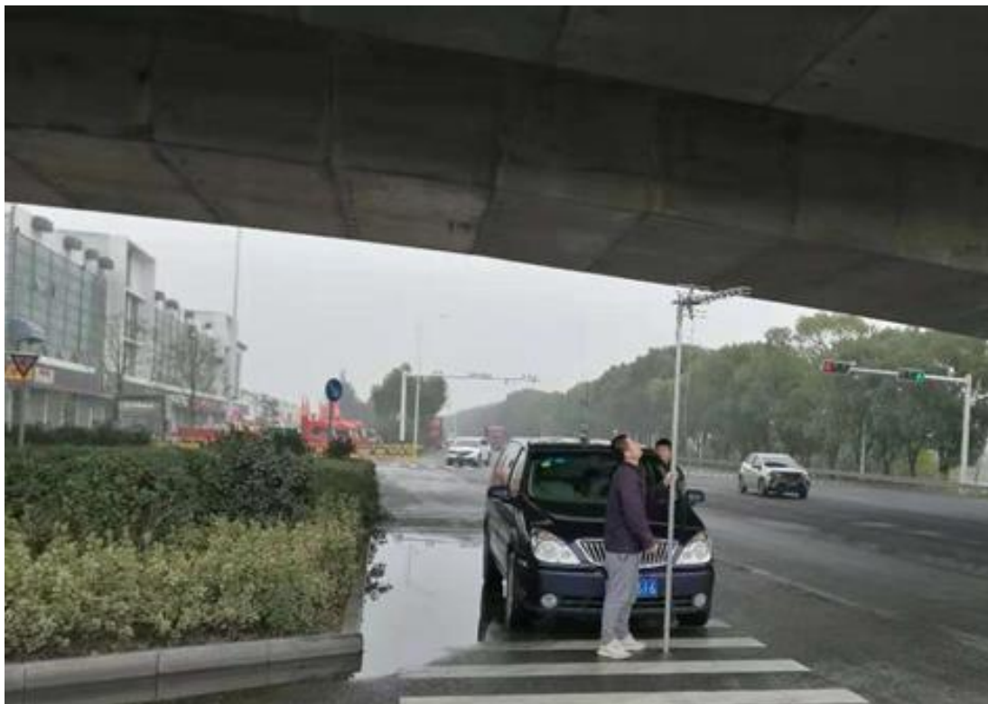
Overpass test point
