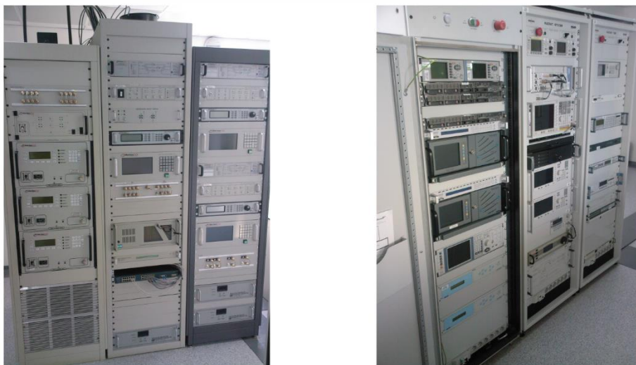
General view of the measurement equipment
