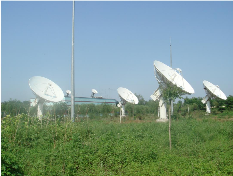
FIGURE 4 Four 7.3 m antennas belonging to System No. 2 and the reference transmitters (on rooftop)
