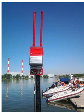
Wireless access station in Rowing Sports Center
