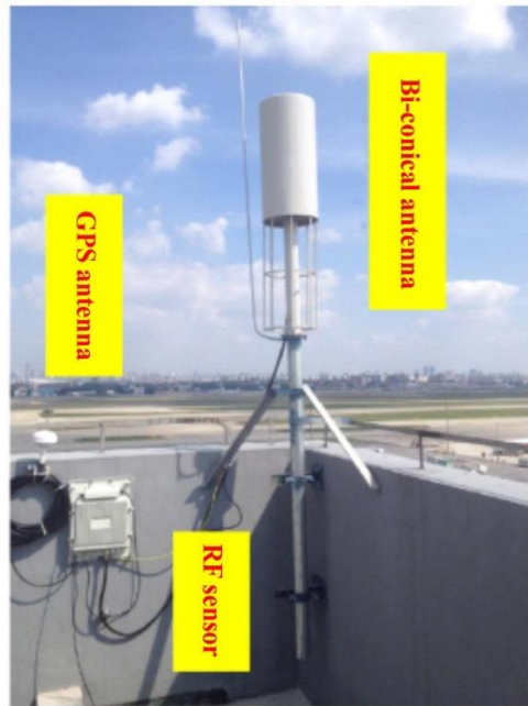
FIGURE A2-6 Cost-effective networkable RF sensor and bi-conical antenna
