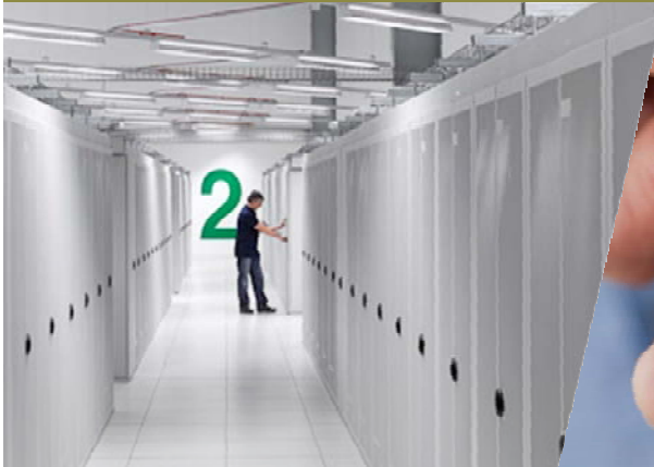
Wynyard Data Center
