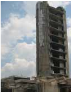
A building destroyed by war Source: ITU/Melissa Arditto.
