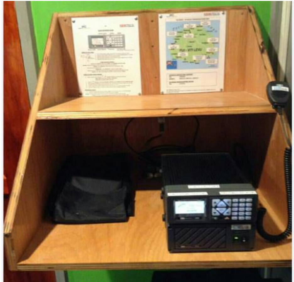
Comms shelf with HF radio at a district office in Fiji
