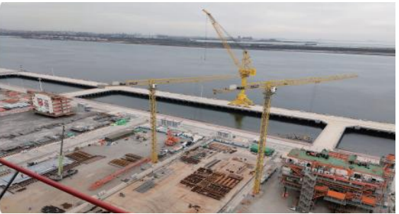
5G+Tower crane monitoring
