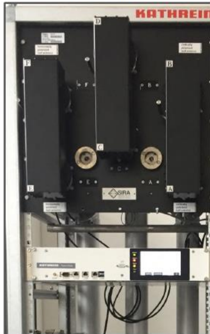
Polarization Switching Unit in Tx room
