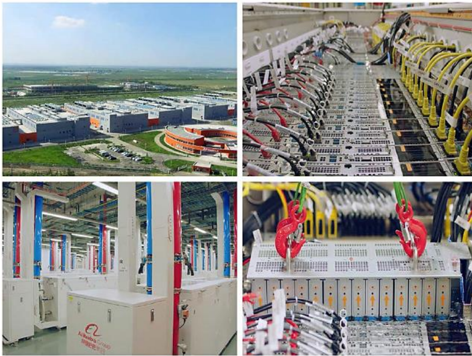
Figure 4. Alibaba Winter Olympics Cloud Data Centre (source: Alibaba)
