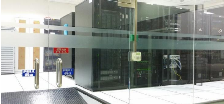
Server room @Chamchuri 9 Building
