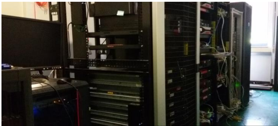
Server room @GIST
