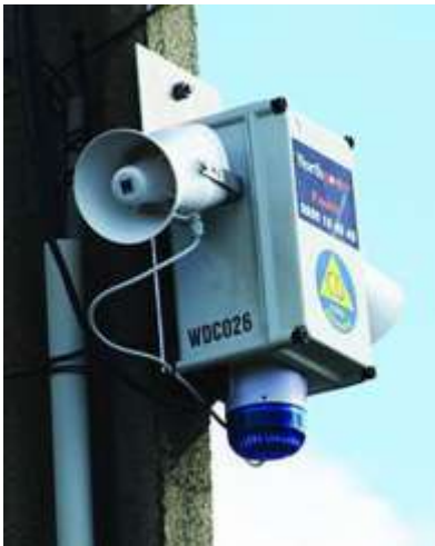
Figure 29 Early Warning Systems: Siren Strobe Photo: Northland Regional Council
