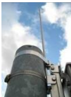
Figure 6 – Air-termination system installed on the top of a mast
