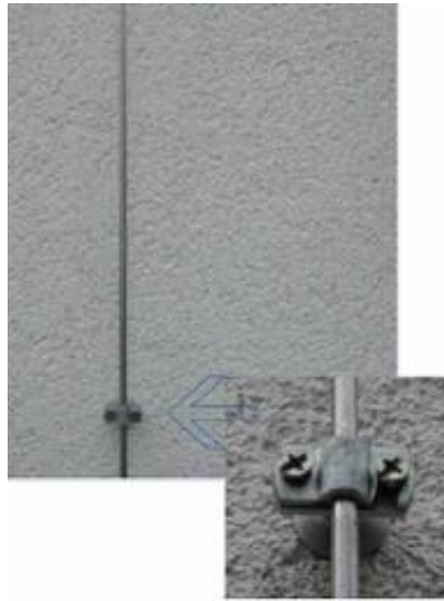
Figure 18 – Down-conductor of a rooftop RBS secured on the wall
