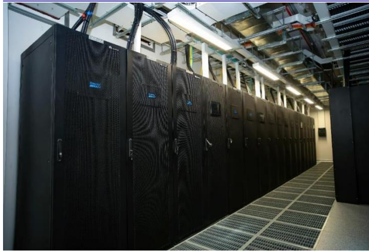
Figure 9 – Smart energy storage system in an edge data centre [b-Huawei]
