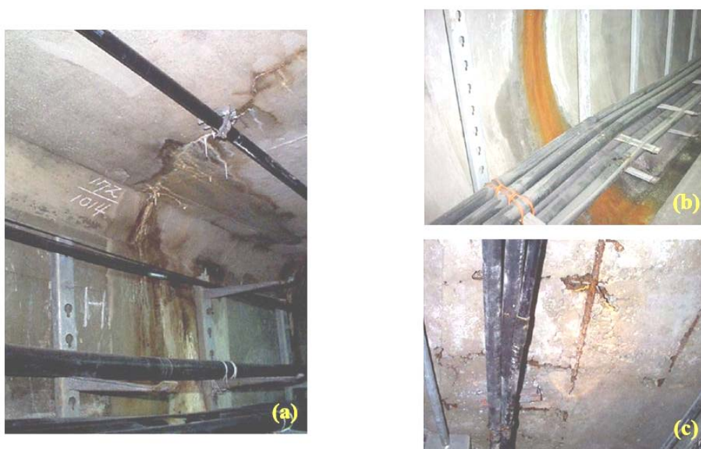
Figure I.1 – Typical deteriorations: a) cracks; b) water leakage; and c) the corrosion of reinforcing steel
