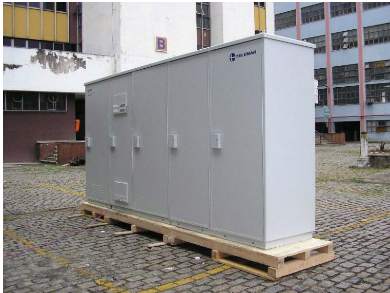
Figure II.4 – Remote access unit (URA)
